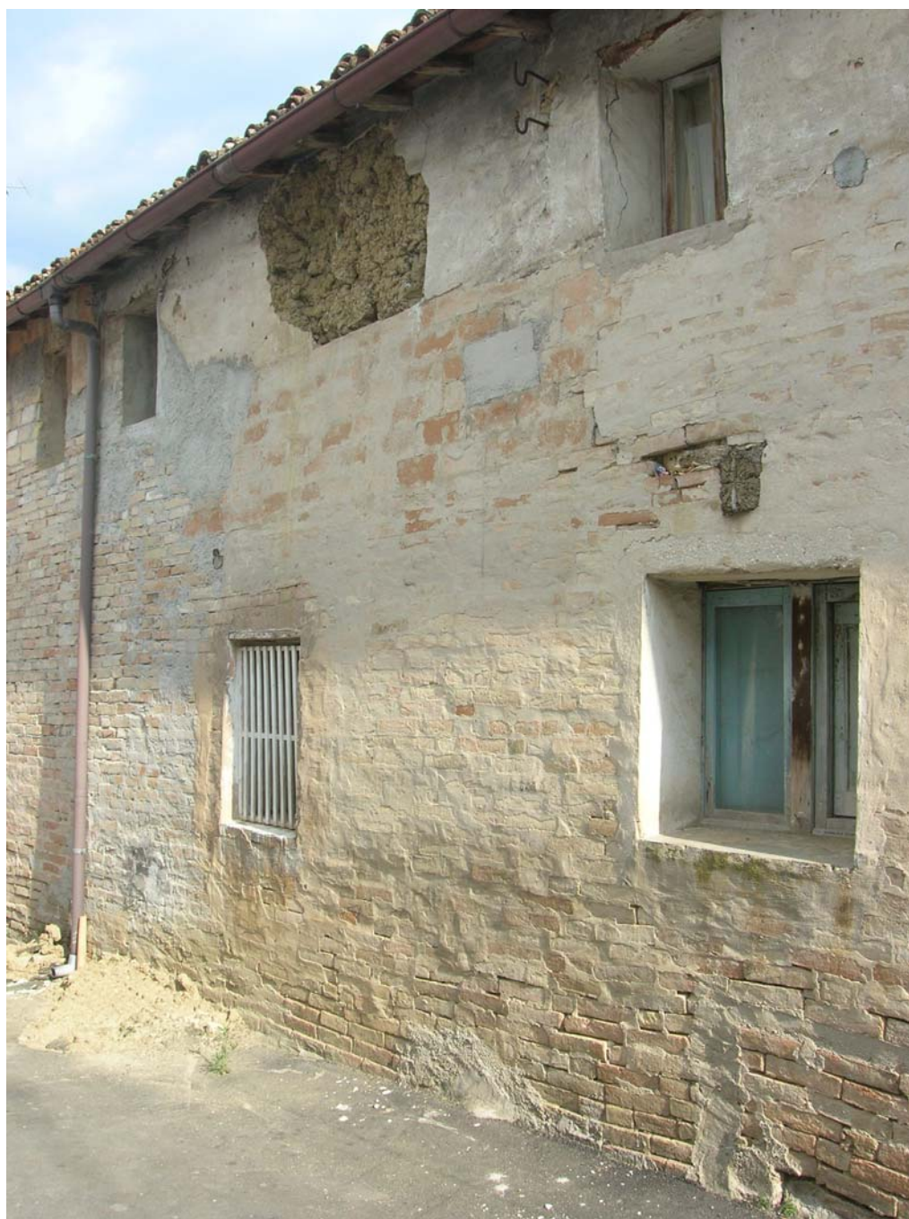
Figure 3. Raw-earth cob walls are often safeguarded by a thick earthen plaster or by a layer of fired bricks.
